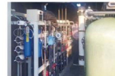
The Pilot Scale Test System of Dongying Sewage Treatment Plant
