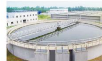
A corner of the Sewage Treatment Plant of Shangqiu Water Co., Ltd.
