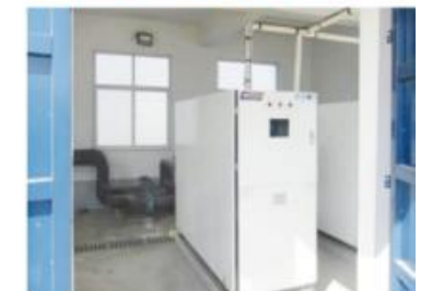
Jiaozuo Sewage Treatment Plant Sewage Water-Source Heat Pump Central Air-conditioning Project
