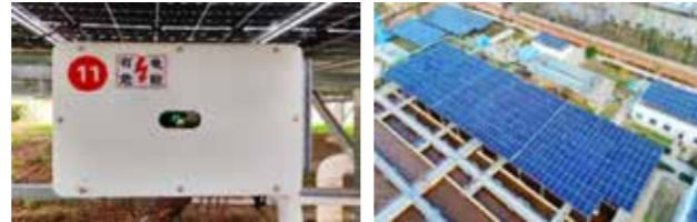
Solar PV Power Generation Facilities
